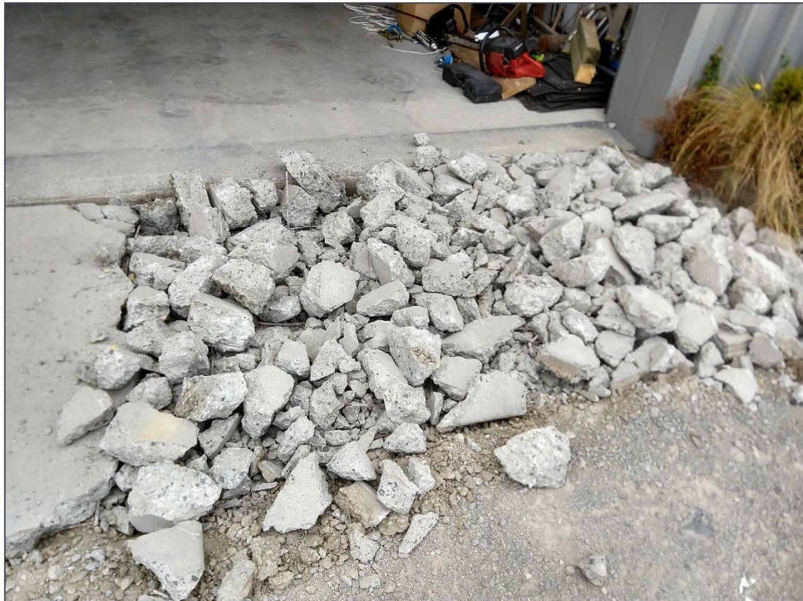
Figure A4: Broken concrete
